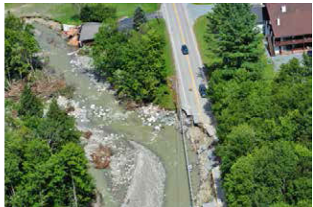
A meander cut through a road (Route 100).
