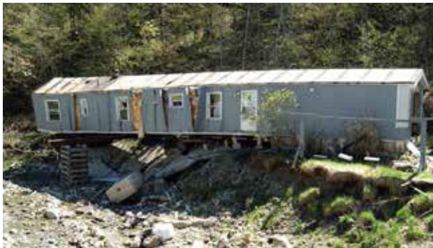
Crumbling house on Flower Brook, near the confluence of the Mettowee River, in Pawlet, Vermont after Tropical Storm Irene, 2011
